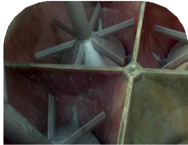
DynaSand® filter modules in concrete basin
